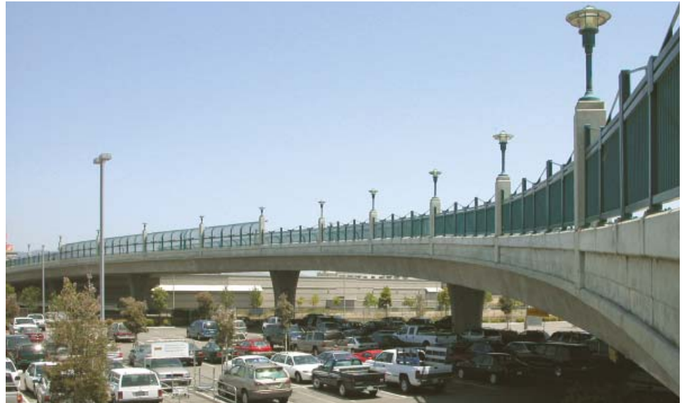
An exterior view of the 40th Street overcrossing's bridge railing and pier-mounted bridge lighting.
